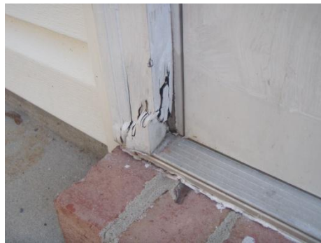
Figure 9 Rear door, damaged /rotten trim
