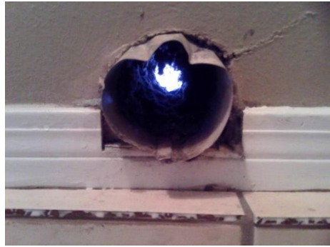
Figure 1 Dryer vent needs cleaning.
