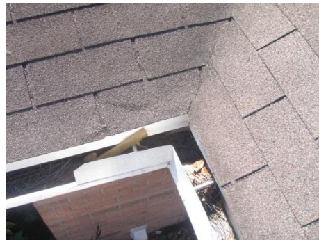
Figure 16 Over Entry, low spot, clogged gutter
