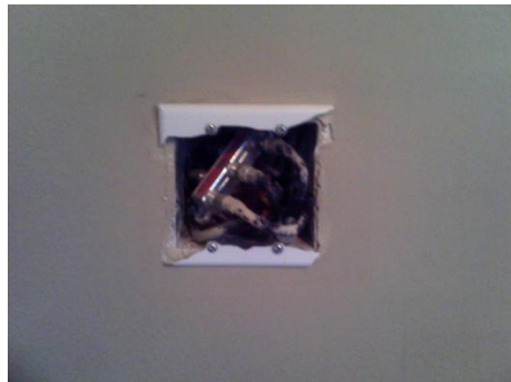
Figure 5 Garage, broken cover
