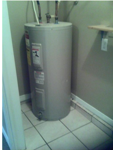
Figure 2 Wtr heater should have catch pan w/drain
