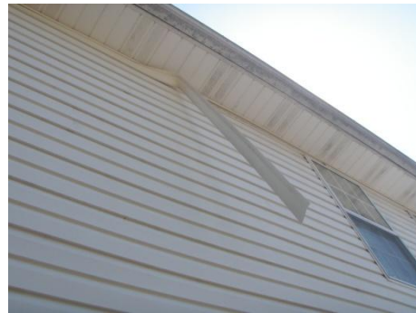
Figure 12 Back of house, Loose siding
