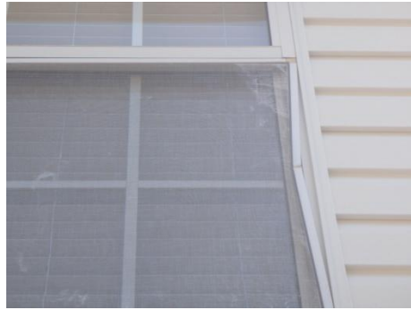
Figure 13 Screens broken, missing
