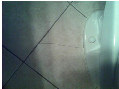
Figure 6 1st floor bath, broken tile.
