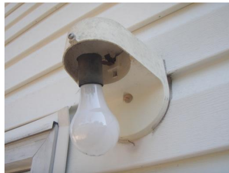
Figure 10 Rear light, damaged
