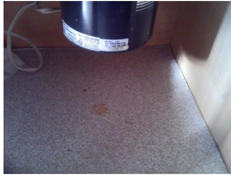
Figure 7 drain leak under disposal.
