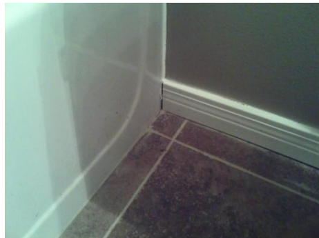
Figure 3 Calking needed at tub/wall area
