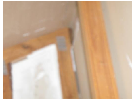
Figure 18 Holes in fire separation
