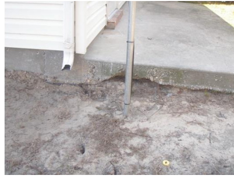
Figure 8 Back fill needed, gutter ext needed
