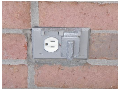
Figure 15 Front Ext outlet, broken cover
